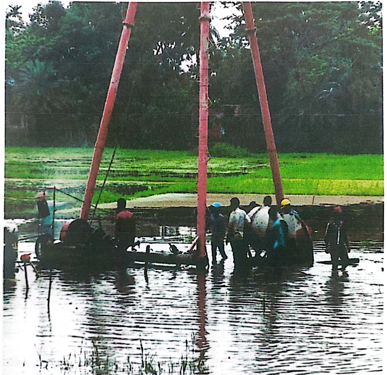
Rooppur, Bogura 400KV Single Circuit Transmission Line
