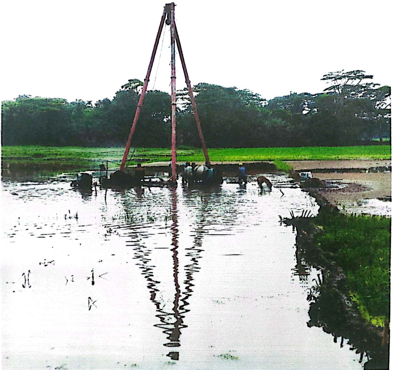
Rooppur, Bogura 400KV Single Circuit Transmission Line
