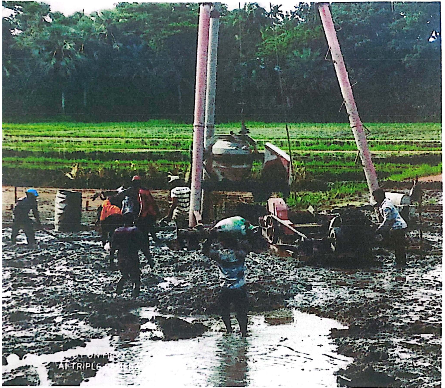
Rooppur, Bogura 400KV Single Circuit Transmission Line
